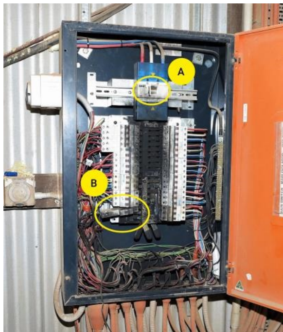
Arc flash damage to the low voltage switchboard showing the isolator in the "On" position (A) and the circuit breaker that was to be removed (B).
