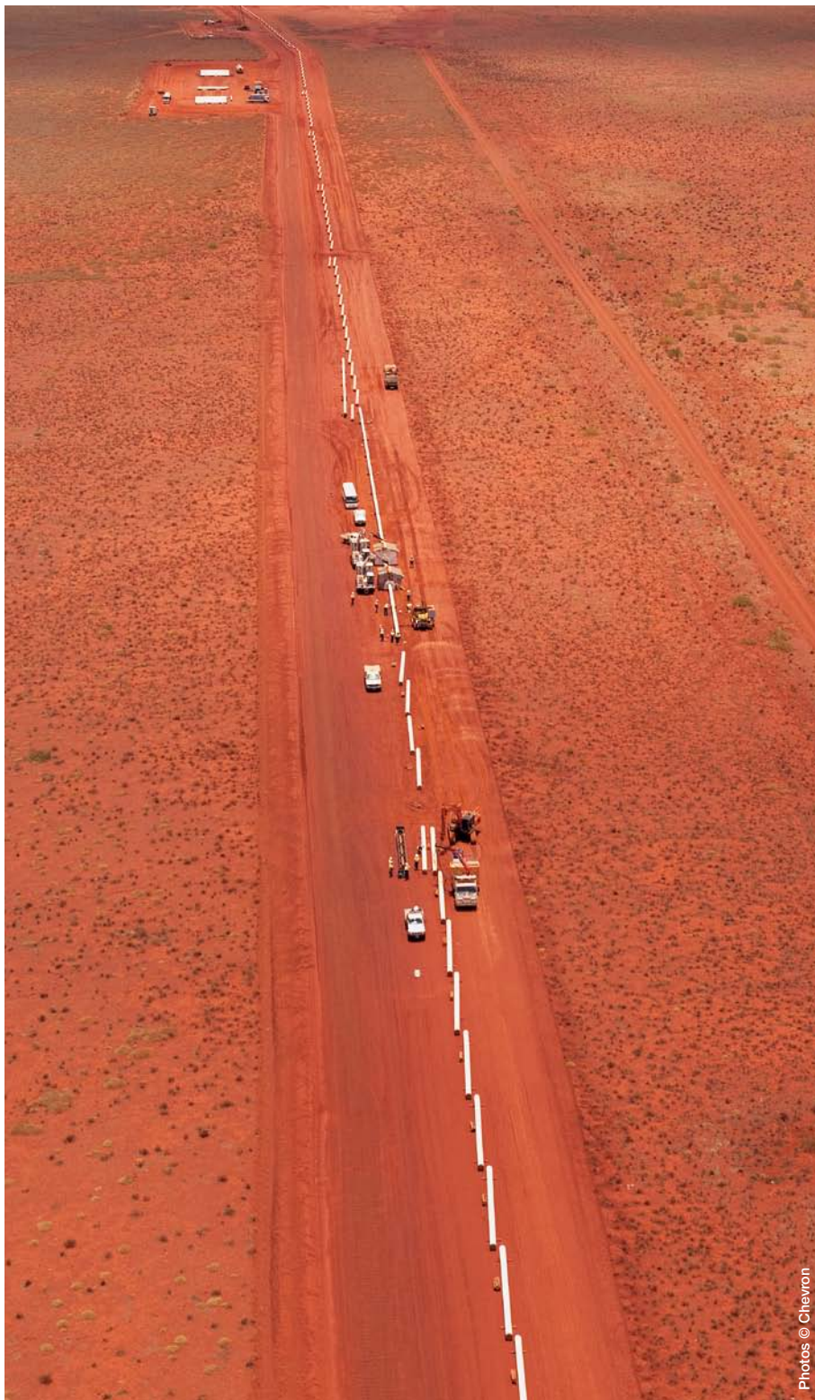
An aerial view of the domestic gas pipeline works on the mainland for the Gorgon gasplant
