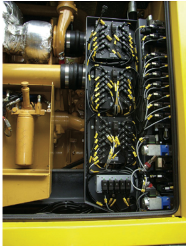
Figure 6.2 Example of turbocharger that has been insulated to reduce the surface temperature and eliminate an ignition source
