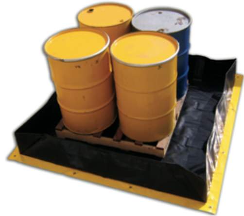
Figure 7.1 Example of bunded pallets
