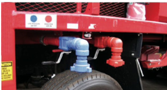
Figure 5.1 Example of engineered compressed air system on an RC drill rig
