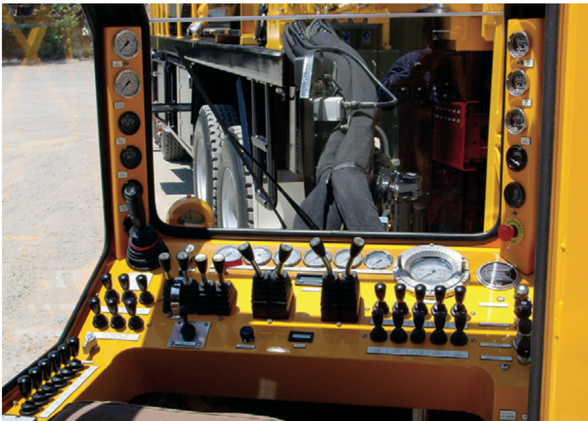
Figure 8.2 Example of hydraulic hoses and electrical cables that are protected and separated with nylon sleeves
