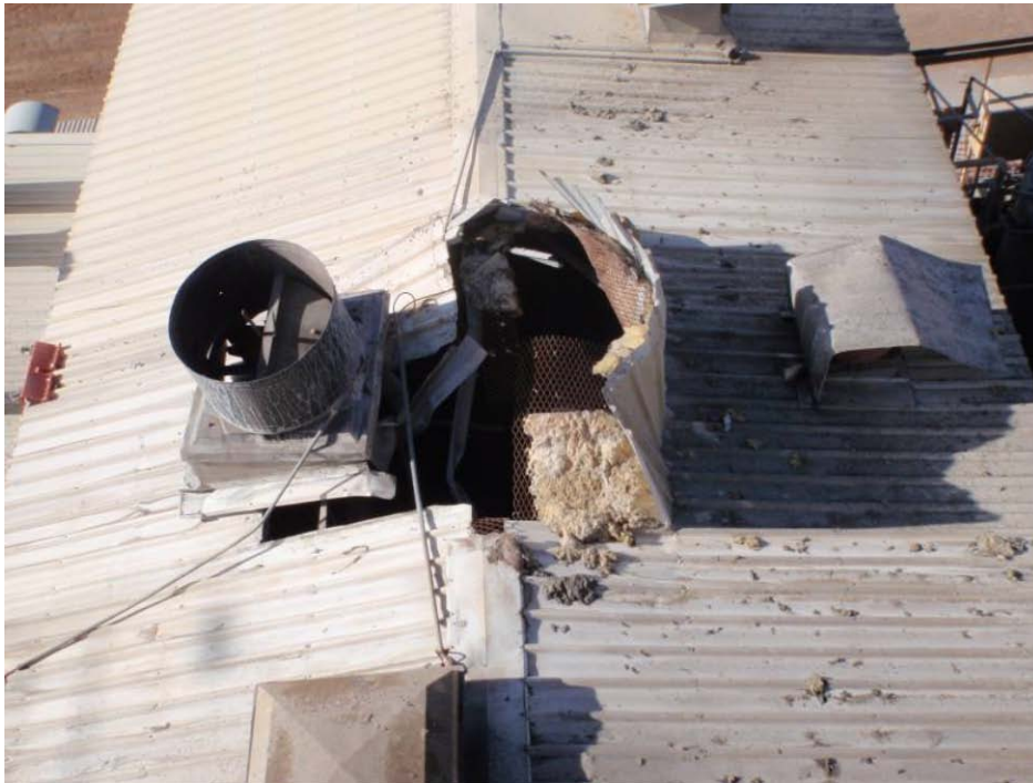
Figure 1 Damage caused when the 500 kg IPSE lid punched through the gold room roof
