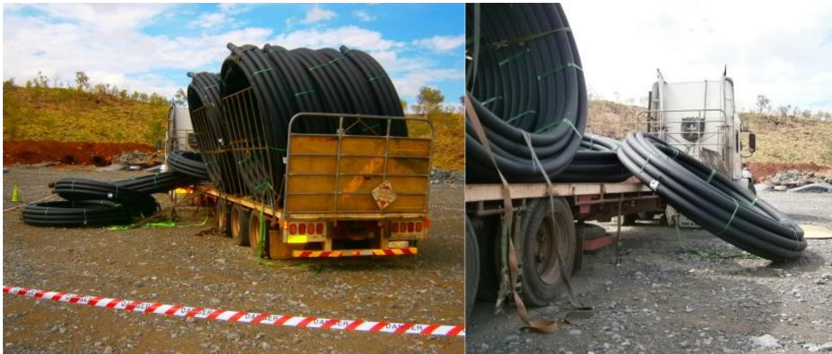
Rolls of poly pipe that fell after the pack's binding strap was cut. The driver fell to the right side of the trailer after being caught in a sliding roll. Note the intact packs of poly pipe rolls at back of trailer showing the arrangement of restraints
