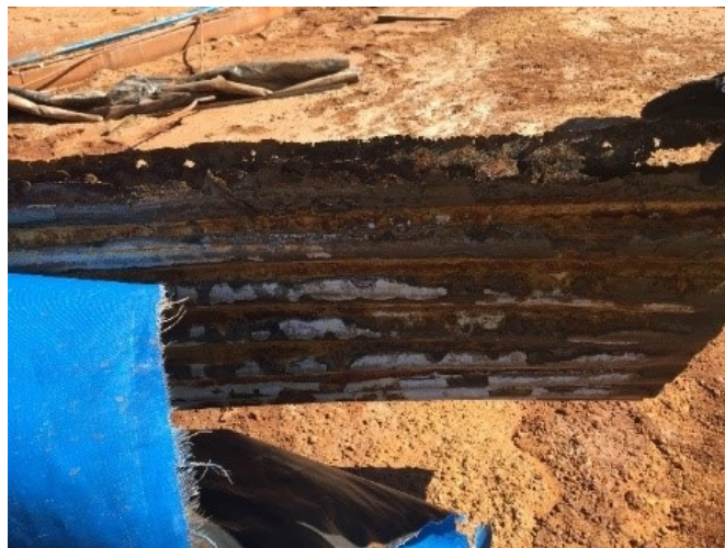
Corroded steel wall of tank
