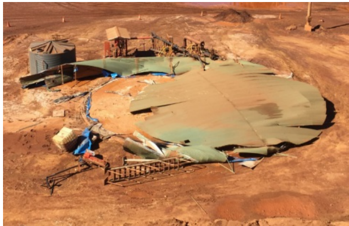
Water tank that failed
