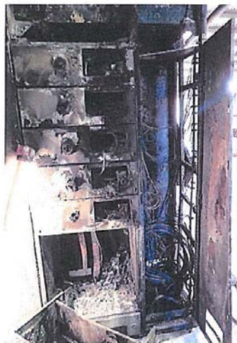
Damaged MCC modules
