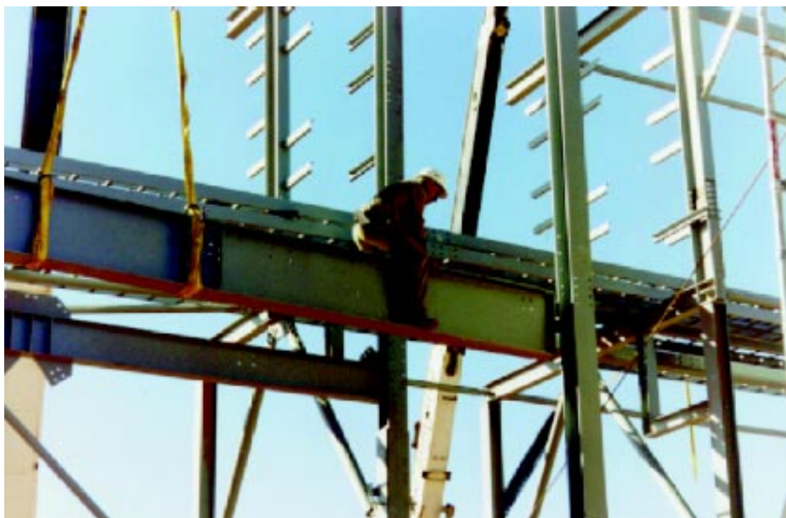
Yes, the beam he is sitting on is suspended from a crane 6 metres above the ground.
